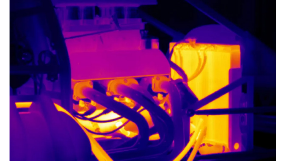
The thermal image of heat building in engine.
